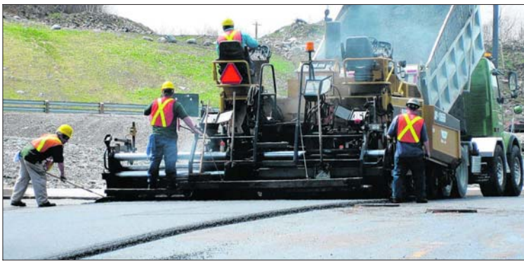
In 2008, almost all of Ocean Contractor's private hot-mix asphalt paving jobs used a percentage of recycled hot-mix asphalt shingle grit product for a total of more than 1,395 metric tonnes.
