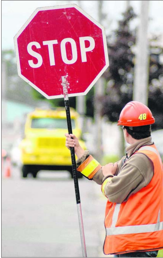
Dealing with traffic still remains the biggest challenge road construction crews face.
