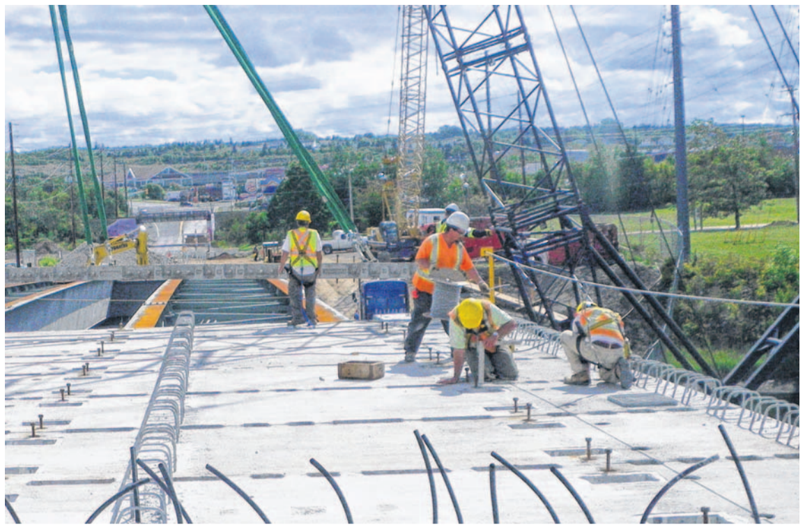
By using precast panels significant cast-in-place concrete formwork can be eliminated, and weather is substantially less of a factor in the project schedule. CONTRIBUTED
