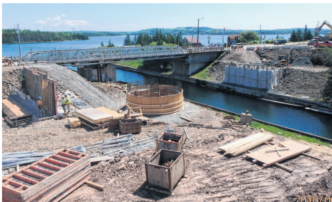
The new bridge is being constructed south of the existing bridge. CONTRIBUTED
