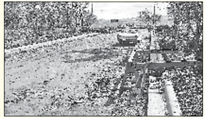
This Oct. 18, 1962 file photo shows the building of an access route linking the Angus L. Macdonald bridge-head in Dartmouth to the Circumferential Highway which funnels traffic down Woodland Avenue. The reconstruction of what was once a narrow dirt road linking the main bridge approach route of Nantucket Avenue to Victoria Road is evident above.
