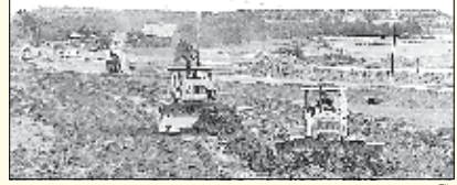
Bulldozers march across level terrain near Truro in this Mar. 7, 1969 file photo as construction crews build a by-pass highway which would link the town with access routes to Trunk 102 and the Trans Canada Highway.
