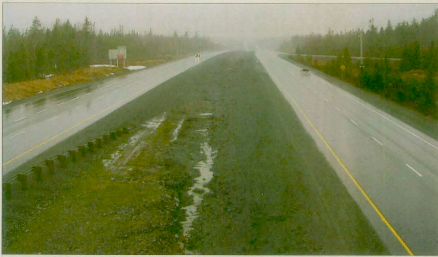
The newest section of twinning on Highway 101 was officially opened last month. Work has begun on the next section of twinning from Ellershouse to Avonport. The project is expected to be complete by 2007-08.
