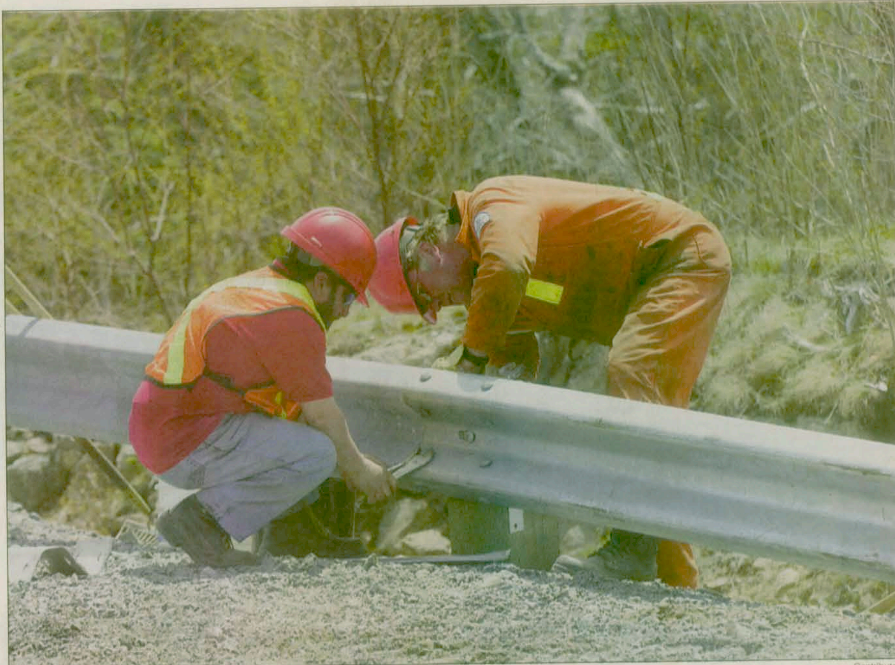
Road workers from Transportation and Public Works repair guard rails near exit 3 on the 103 highway in Halifax County May 12.
