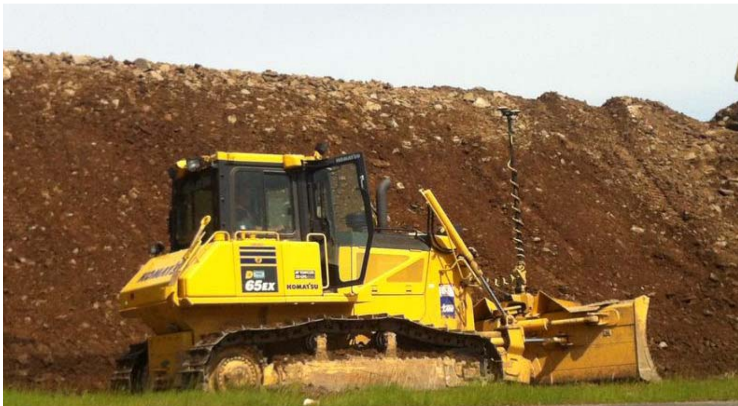
Using machine control on excavators has helped Alva Construction Ltd. improve production in some cases as high as 25 to 30 per cent.
