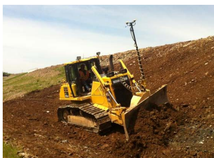
Alva Construction Ltd. has helped outfit their excavators with GPS technology, provided by On-Grade Inc. in Dartmouth.
