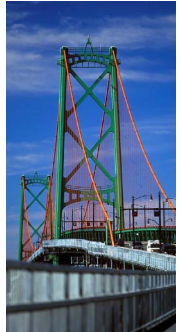
The Macdonald Bridge Suspended Span Redecking Project is expected to be completed in 2016.
