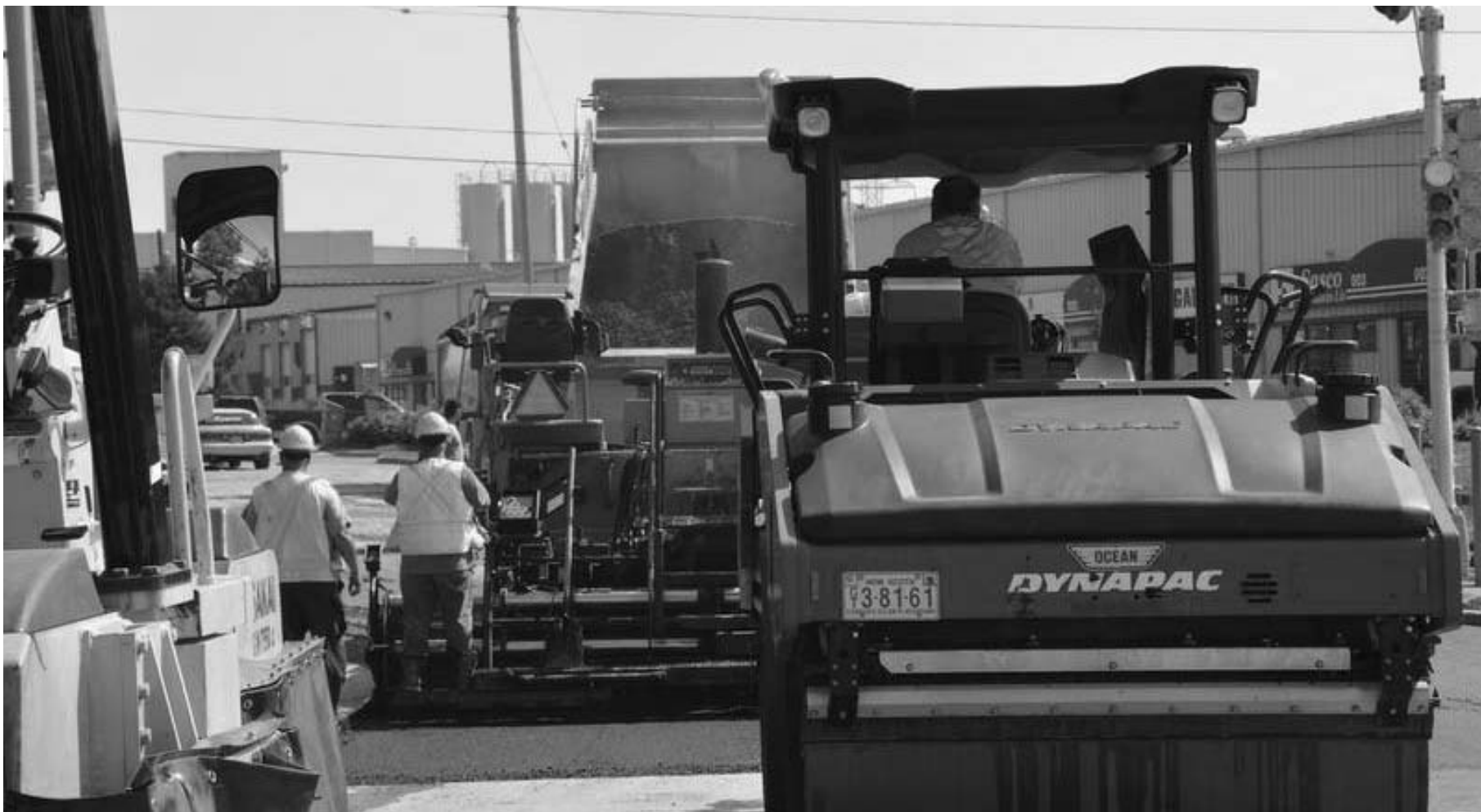
Road building is one of the longest standing and most successful industries in Nova Scotia, with a storied history going back more than 100 years.
